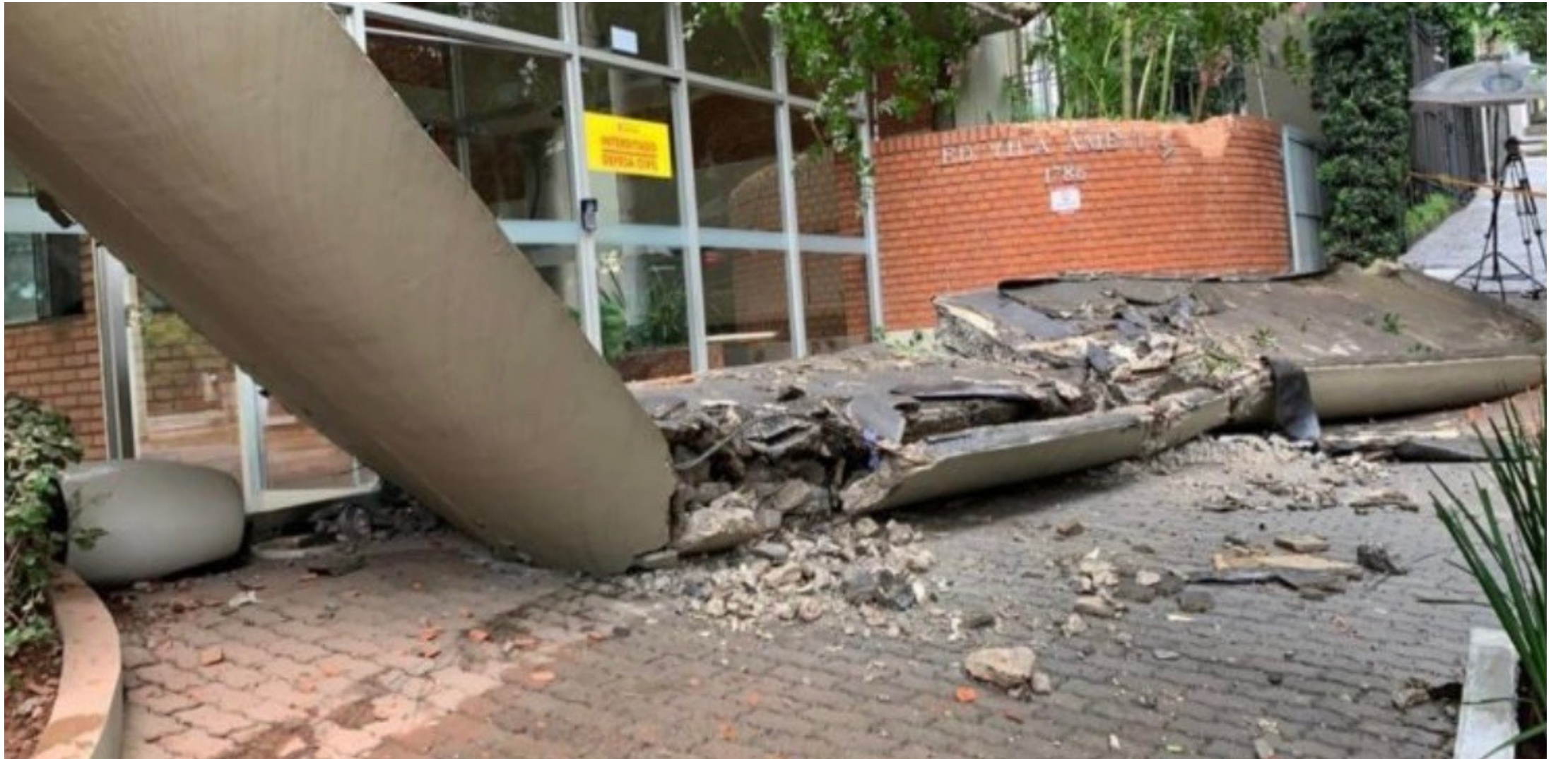
Colapso marquise ( São Paulo/ SP)
